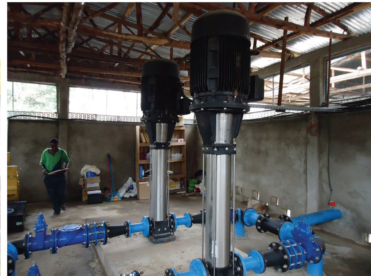
Jewi Permanent Water System, Gambella Regional State
